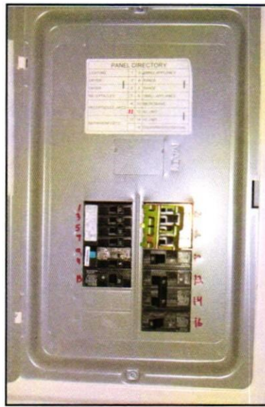
Circuit Breaker Panel
