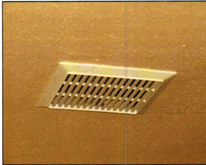
Typical Bathroom Exhaust Fan
