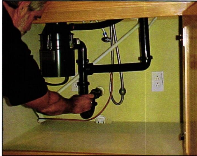
Garbage Disposal Under Kitchen Sink
